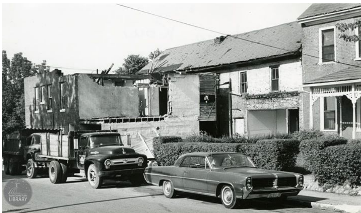
The Fisher Row Houses undergoing renovation. Either One Richardson's house is on the right, and that may be his automobile parked in front.
